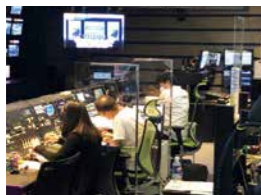
The sub control room is also partitioned with acrylic panels
